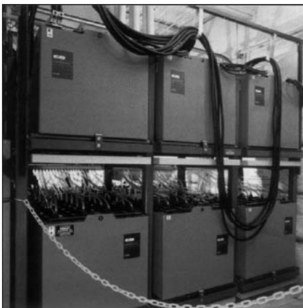
Figure 6 Large lead-acid battery bank
